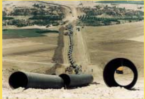
Construction of the EIB-funded Maghreb-Europe gas pipeline from Algeria via Morocco to Spain
