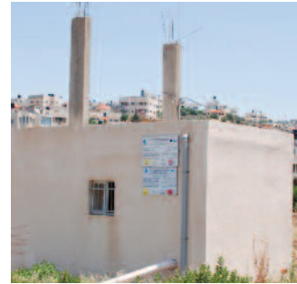
One of the projects of well rehabilitation in the Qabatya locality, district of Jenin.
